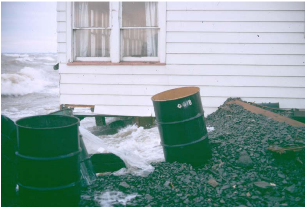
Example of structural damage to a home foundation due to wave forces
